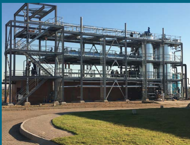
The eutectic freeze crystallisation (EFC) unit designed and built by Prentec at the Tweefontein Colliery in Mpumalanga, based on research done at UCT's chemical engineering department. Much of the research was funded by the Water Research Commission.
