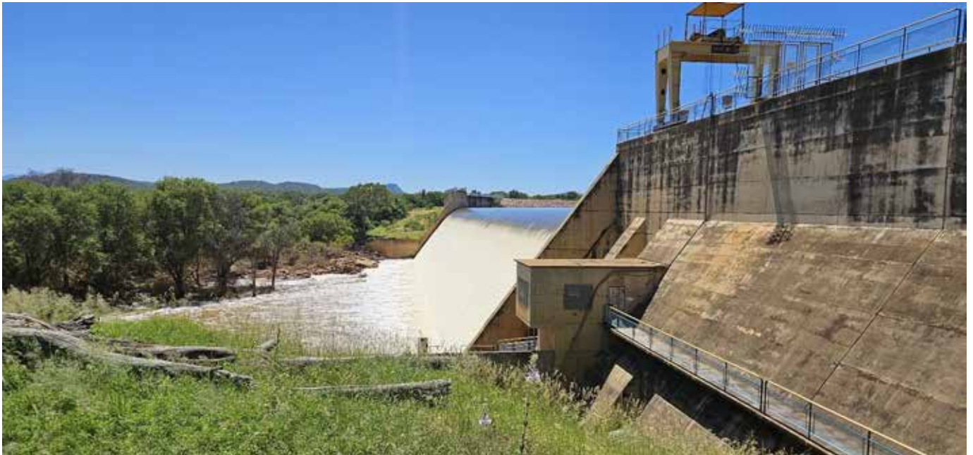
A view from the dam wall of the Glen Alpine Dam wall in January 2025. This rapid increase in water levels facilitated the recovery of fishery resources with a marked increase in species abundance and diversity.
